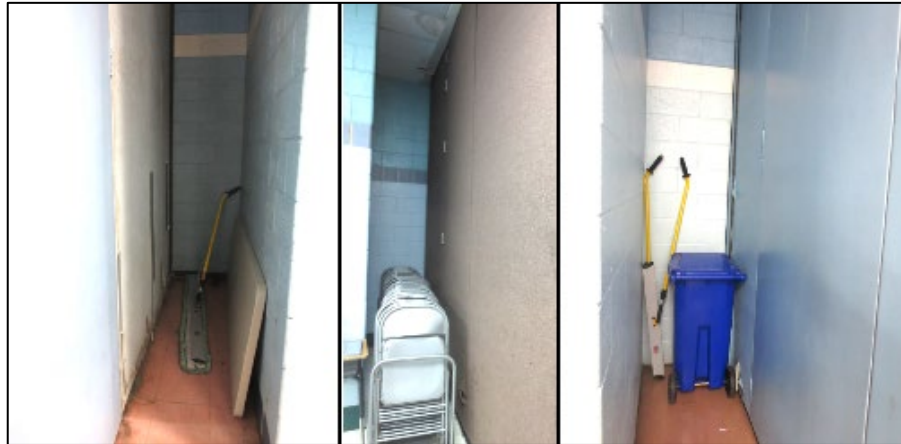
Figure 10: Electric Horizontal Retractable Partition pockets misused for storage
