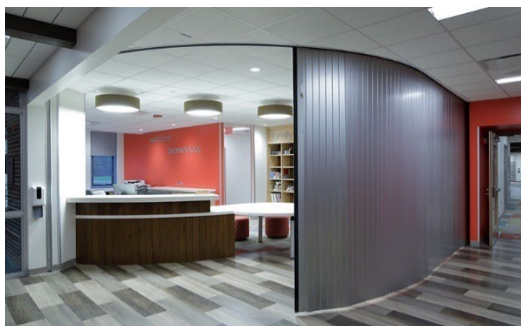
Figure 2: Electric Horizontal Coiling Door
